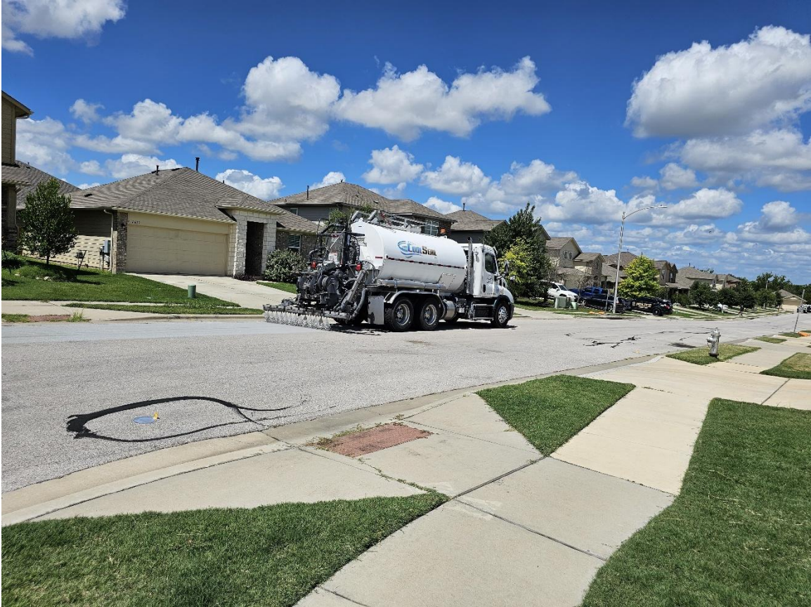
Figure 2. An image of the application process of Cool Seal by Guard Top. You can see the reflective pavement coating being sprayed on the pavement out of the back of the distributor truck.
